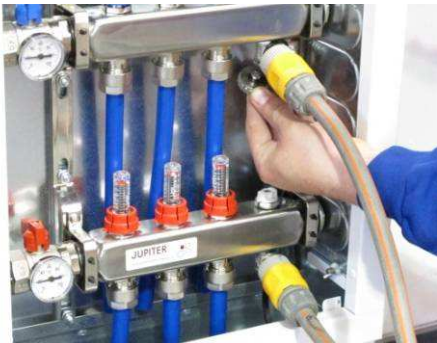
Once purged with air close fill & drain valves using cap. Close upper return valve first then lower fill valve. Only then turn off water supply and remove hoses.
