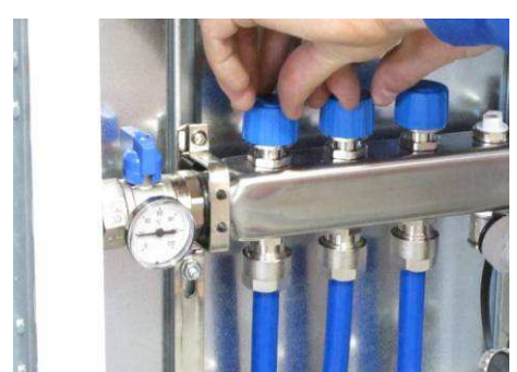
Once no more air bubbles emerge, simultaneously close the completed circuit and open the next one.
