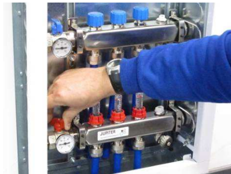
Close isolating valves
