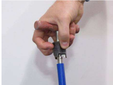
Always calibrate the end of pipe with bevelling tool before attaching to manifold
