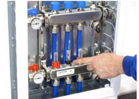
Ensure all flow meters are open by removing red cap and turning anti-clockwise
