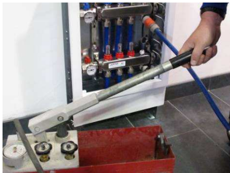
Once connected pump up to 8 bar. Once satisfied that there are no leaks, leave on test for a minimum of 1 hour.
